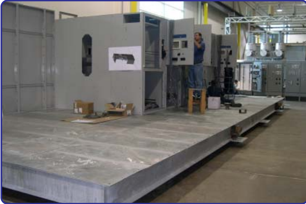
25kV Type C Arc Resistant Switchgear In a House, Switchgear Being Assembled on House Base—House Walls Being Placed
