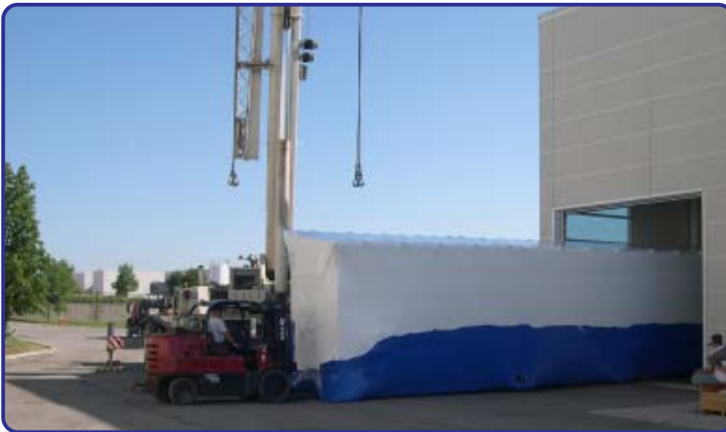
25kV Type C Arc Resistant Switchgear In a House, Switchgear Section After Shrink Wrapping—Being Moved Out For Loading
