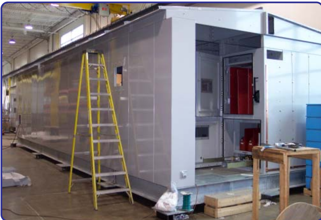
25kV Type C Arc Resistant Switchgear In a House, Aisle & Switchgear Section Connected—Load Break Sw Cell Seen on Right
