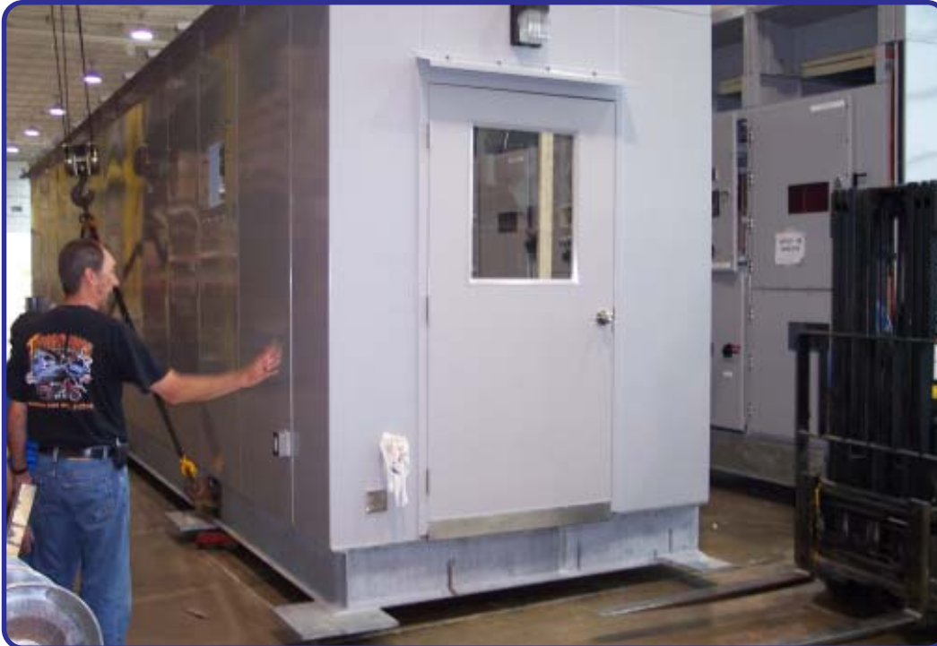
25kV Type C Arc Resistant Switchgear In a House After Factory Commissioning—Aisle Being Separated For Shipment
