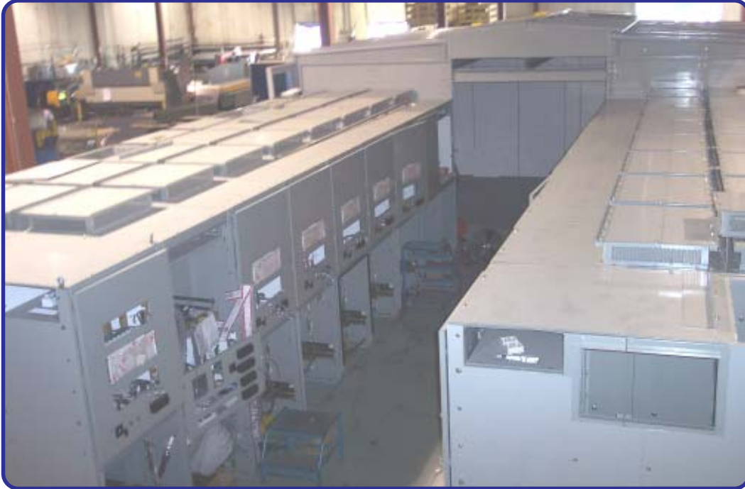
15kV Type C Arc Resistant Switchgear in a House Being Fully Assembled in the Factory- Switchgear Line Up, Control Area
