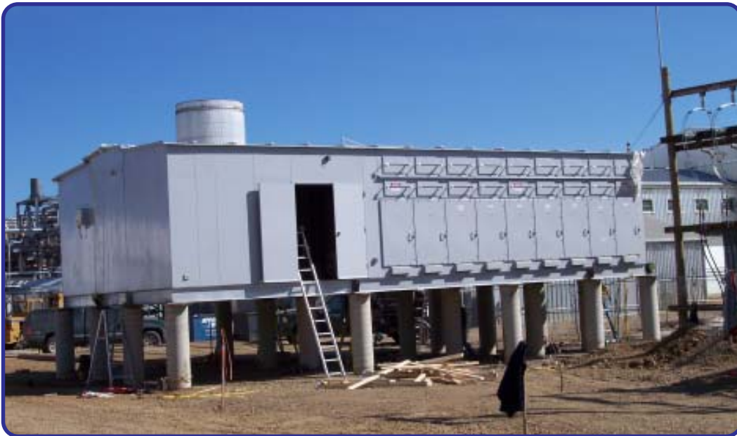
15kV Type C Arc Resistant Switchgear In a House Three Shipping Sections Fully Assembled at Site 3000 miles later
