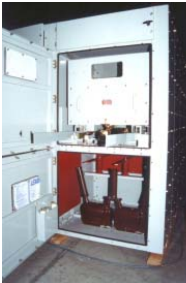
Arc-Resistant Switchgear PT Compartment
