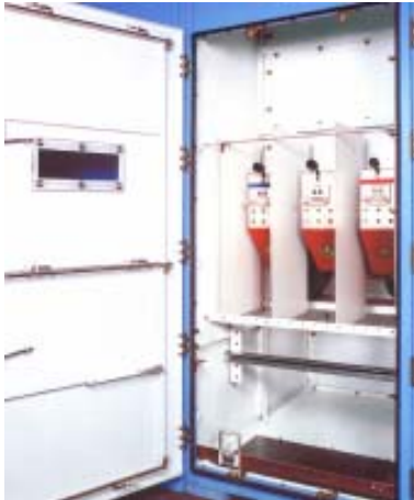
Arc-Resistant Switchgear Cable Compartment
